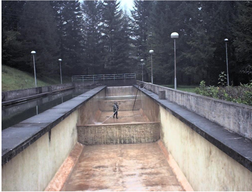
Figure 5: Potable water treatment plant Tilava – washing out of sedimentation tank
