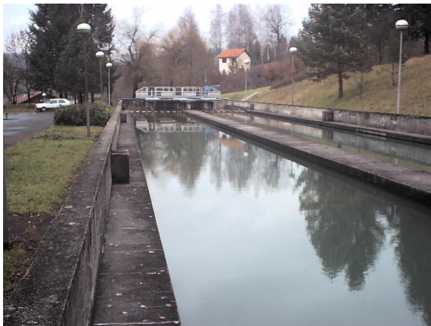
Figure 4: Potable water treatment plant Tilava – sedimentation tank
